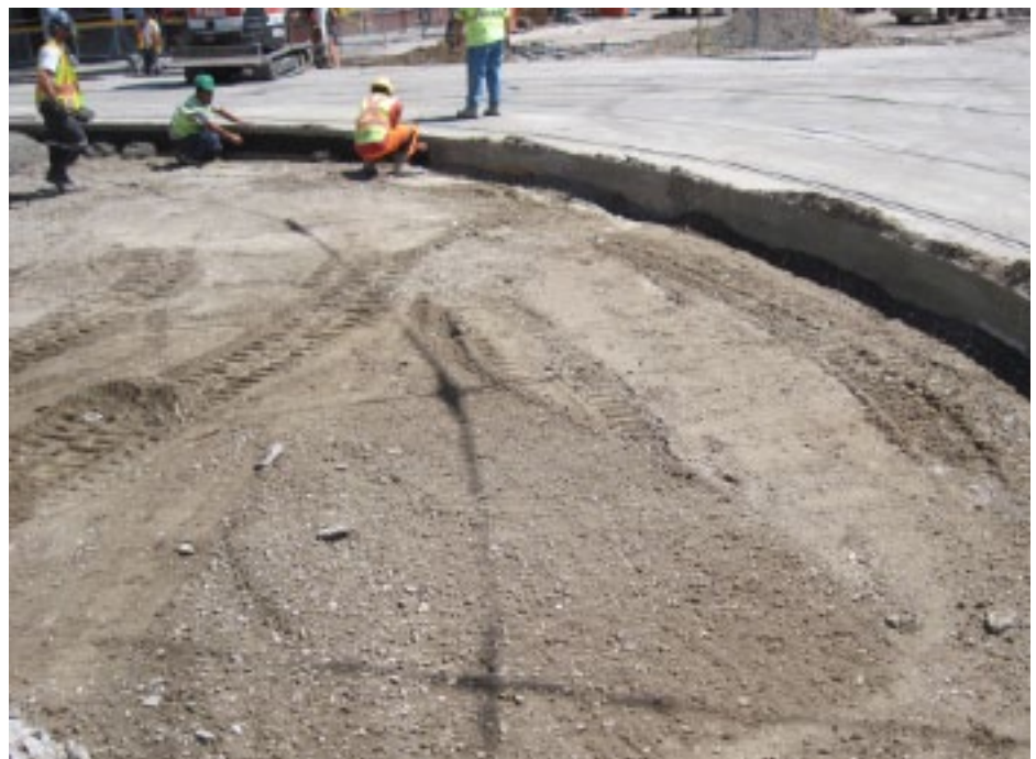
Recycled aggregate being applied at an ongoing project at Queen St. and Spadina Ave. in Toronto. Recycled concrete was used under the track foundation slab and under the concrete road base as a Granular A base.
